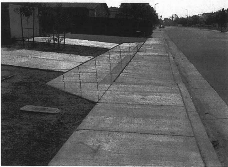
Driveway without rolled curb & gutter
