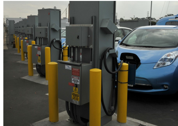
Figure 35. Examples of industrial-grade electric vehicle charging stations. Expensive retrofits will not be necessary if planned into the site. Electric vehicle fleets reduce lifetime cost. (U.S. Air Force photo/Sarah Corrice)
