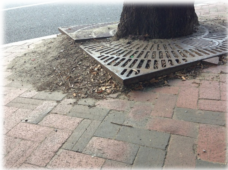
Figure 5-3: Tree well with metal grate raised by root growth in Richmond, VA (Source: SeeClickFix)
